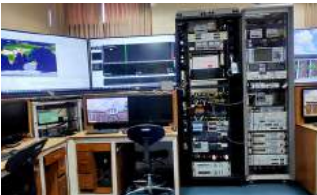
IIST Satellite Ground Station Control Room
